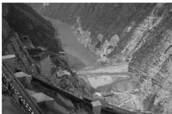
Figure 9 Photograph of the construction site of Jinping II hydropower station in China.
